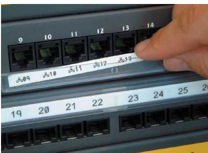
Punch block & patch panel labels
