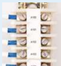
Terminal block marking
