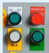
Control panel labelling
