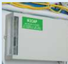
Control panel labelling
