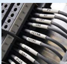
Wire & Cable Marking
