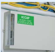
Control Panel Labelling
