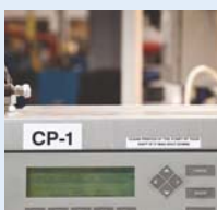
Control Panel and Electrical Panel Labels
